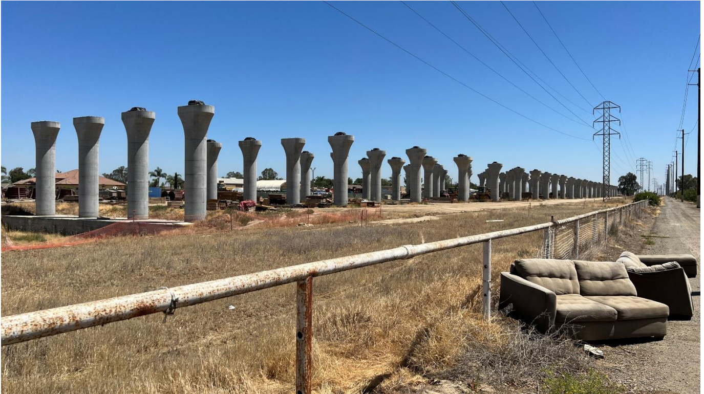
Photo 7: View of California High-Speed Rail construction adjacent east of the Subject Property.
