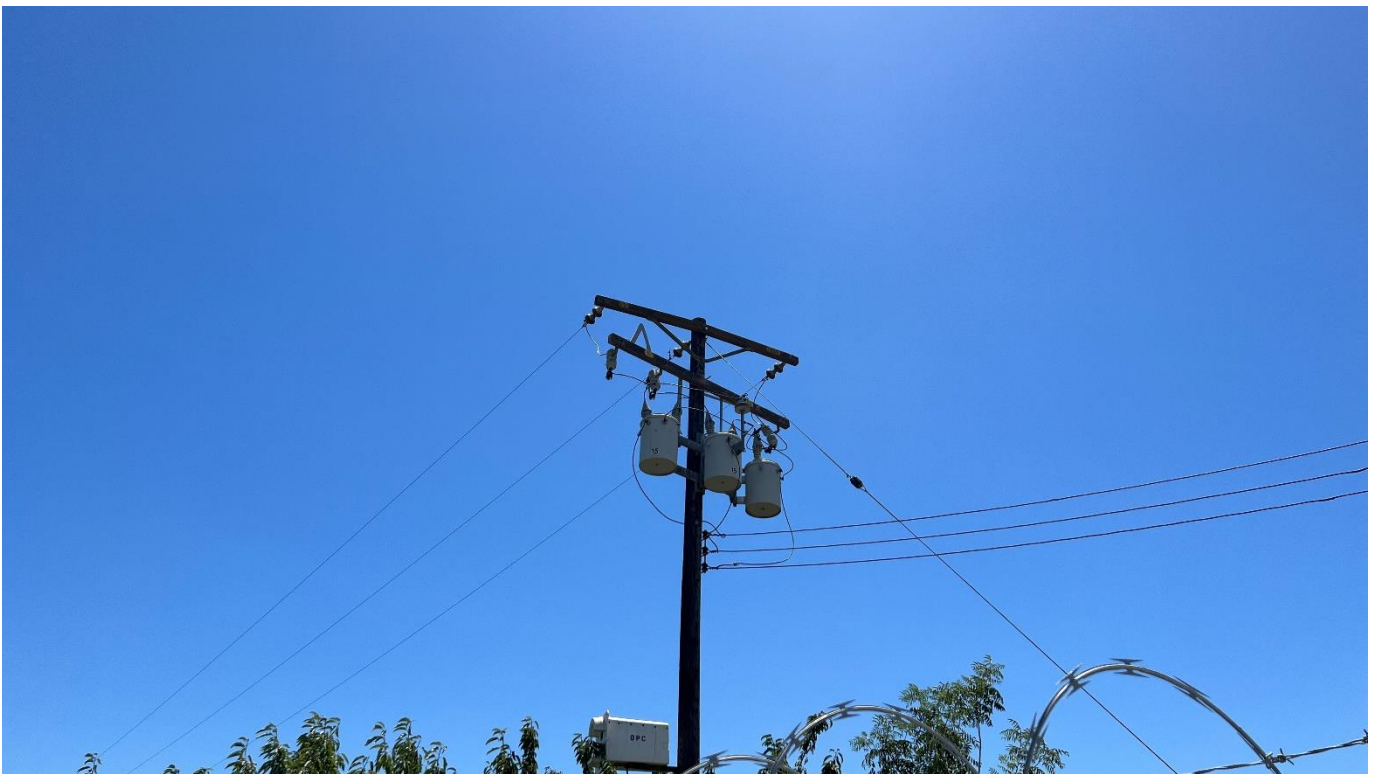
Photo 2: View of pole-mounted transformer along western boundary of the Subject Property. BSK did not see evidence of staining or release from the pole-mounted transformer.
